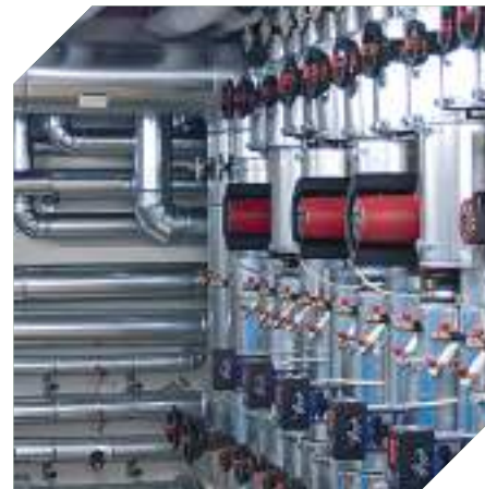
Sanitary hot water
